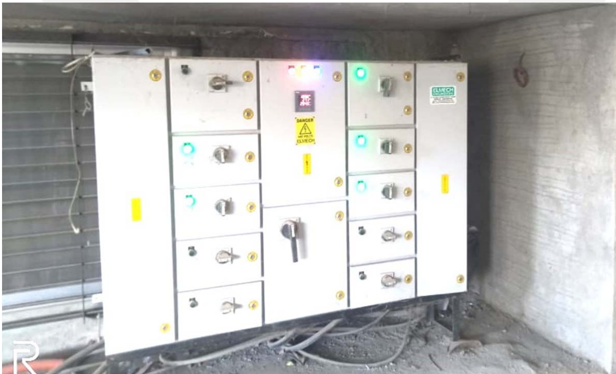
High Speed Diesel Generator (HSDG)
