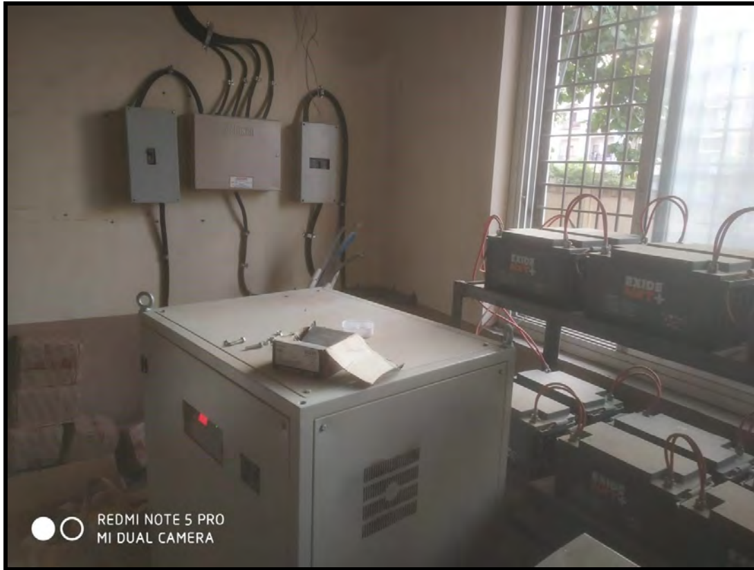
Power Backup UPS room
