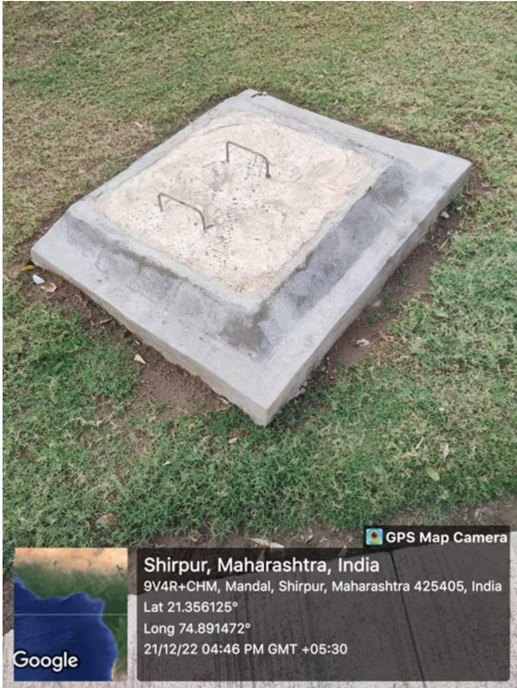
Figure 18 Rain Water Harvesting Point
