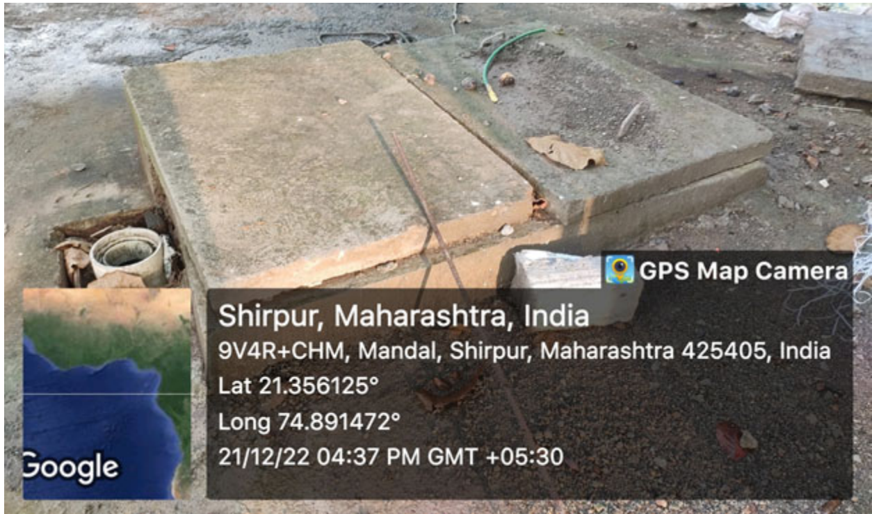
Figure 20 Water Tank at College
